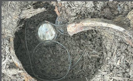
Example of a covered water meter
