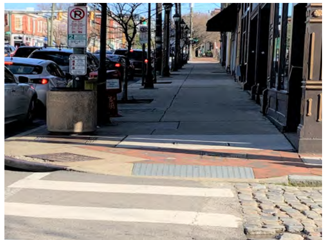
Examples of damaged and missing sidewalks and inconsistent materials
