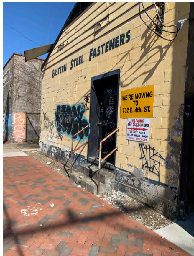
Example of blighted buildings that have a negative impact on the appearance of the area
