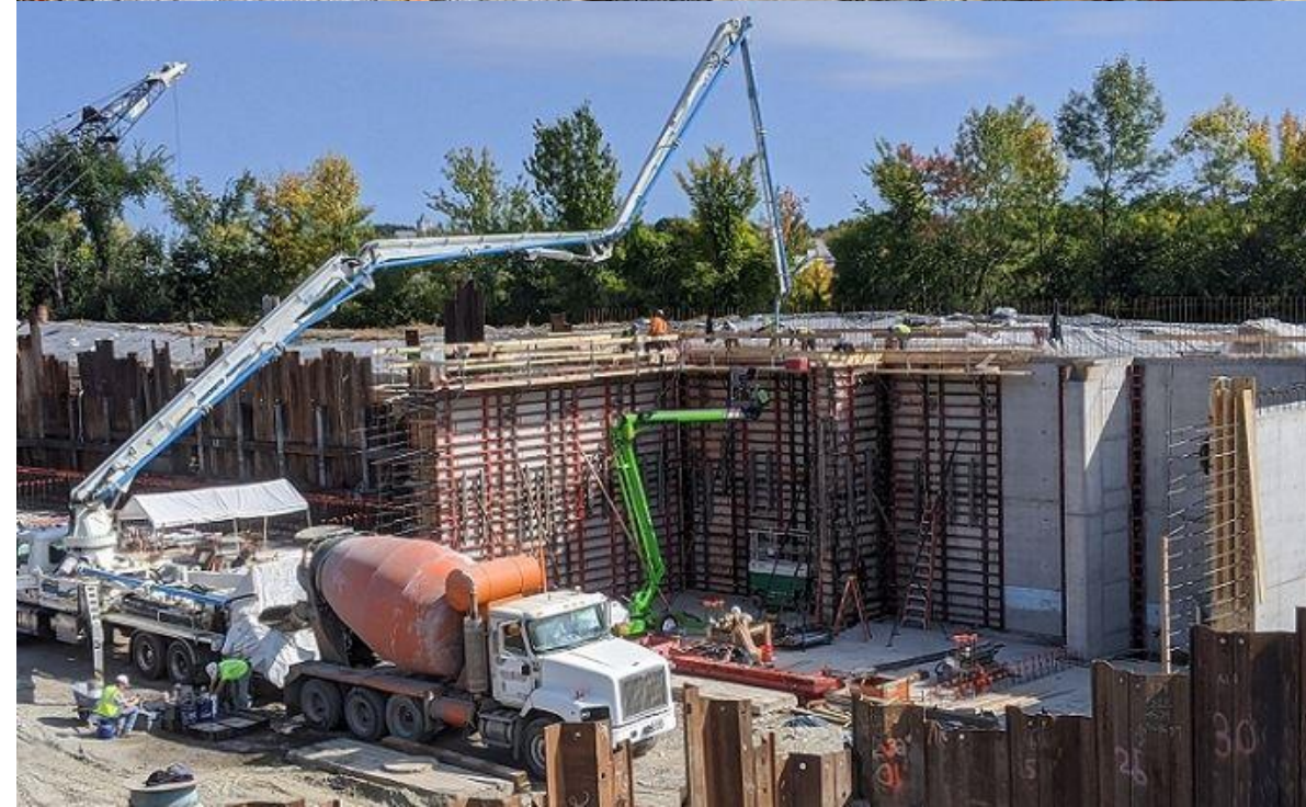
Photos of Davis Brook CSO Storage Tank | Bangor, ME
