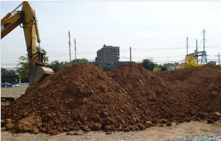
No Stockpiling of Excavated Materials
