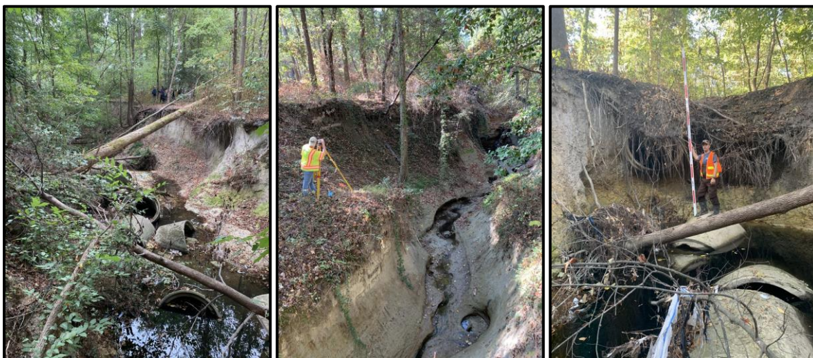
Figure 4-13. Pre-restoration condition of Pine Camp Creek stream channel.
